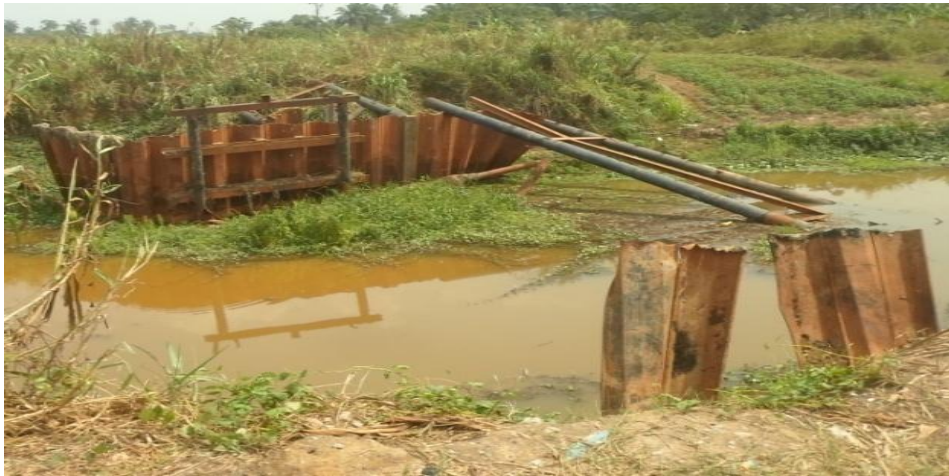
Figure 2. Rusty and Dilapidated Iron Bridge in the Kolo Creek.
