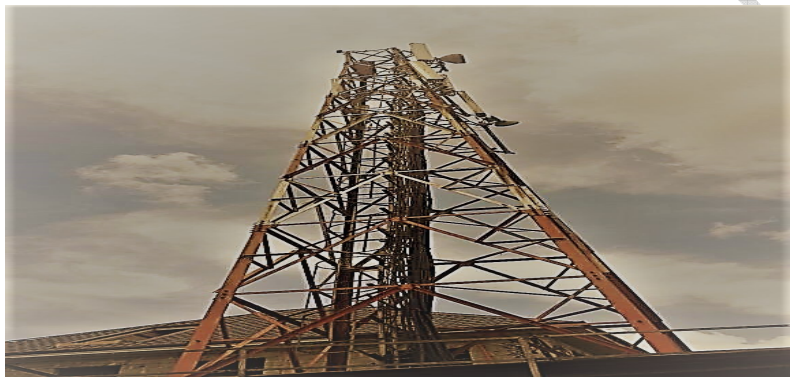
Figure 1. Picture of MTN Mast visited at Rumuolumeni
