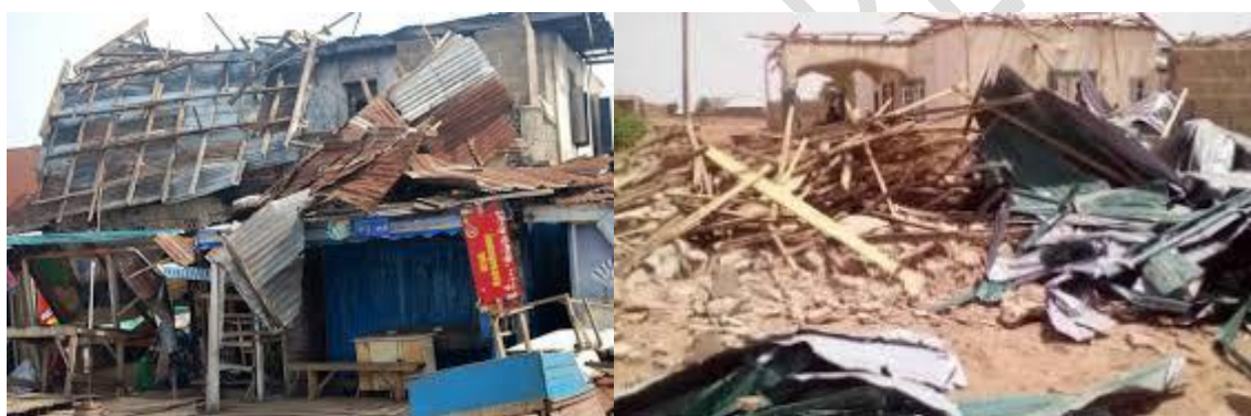
300 301 Fig 10: Damages done in Wukari
