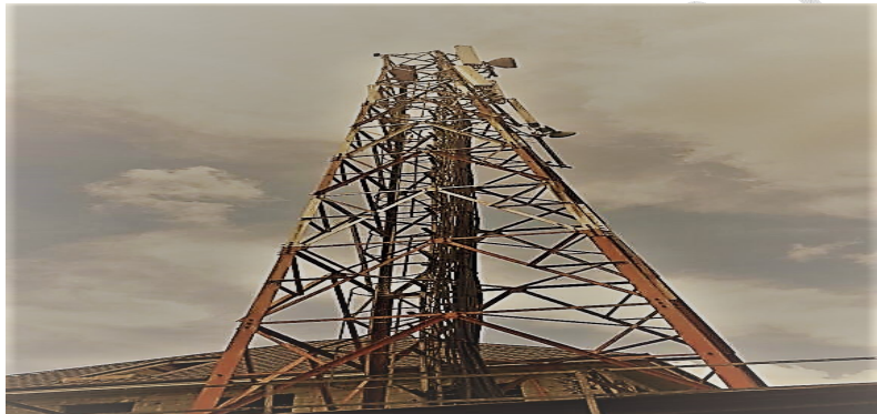
Figure 1. Picture of MTN Mast visited at Rumuolumeni
