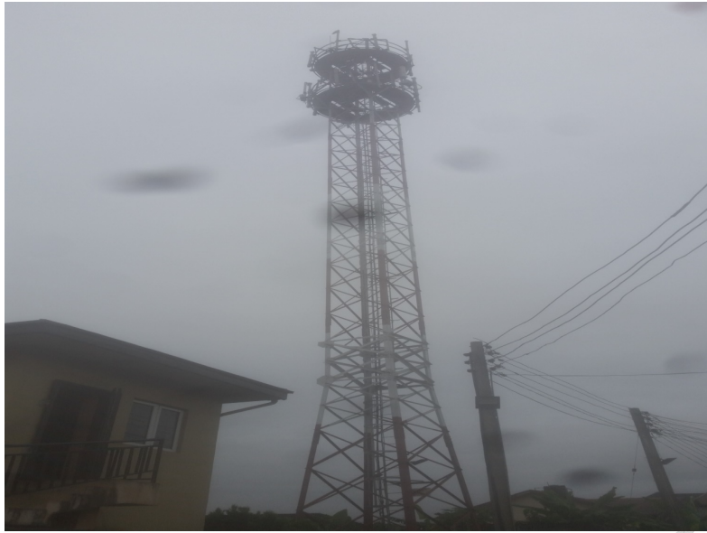
Figure 2. Picture of Airtel Mast Visited at Akwaka
