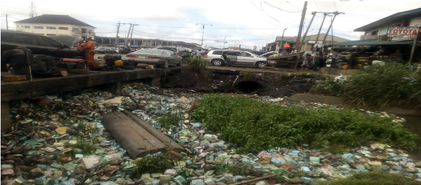
Plate 3: Blockage of water channel with assorted (especially Xenobiotic) waste products associated with anthropogenic activities around the creek in Port Harcourt
