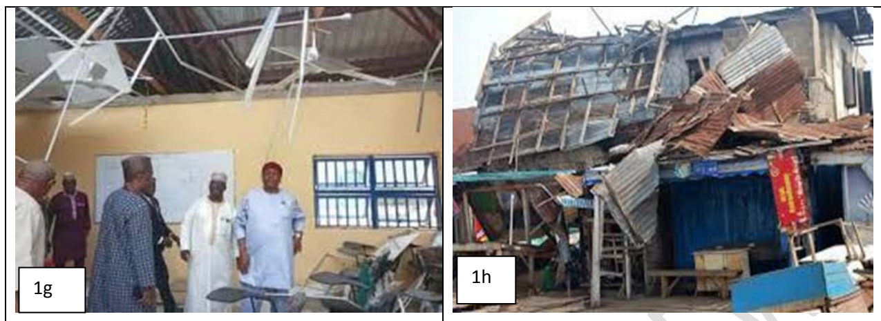
190 Fig. 1a-g showing Damages caused by Rainstorm on 5 th May, 2018 in (1a) Nigeria Television 191 Authority (NTA) Jalingo Office (1b) National Youth Service Corps Camp Jalingo (1c) Class 192 room blocks of Government Model Day Secondary School Jalingo (1d) ICT laboratory at the 193 Government Science Secondary School Jalingo (1e) NCCF Family House Donga Road Jalingo 194 (1f) Lecture Hall at Taraba State University (TSU); (1g)The Vice Chancellor of TSU shows the 195 extent of Damage to the Visitor of the University, the Governor of the state and (1h) Wukari 196 town
