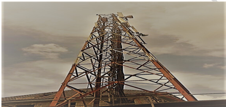
Figure 1. Picture of MTN Mast visited at Rumuolumeni
