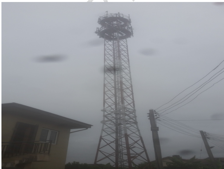
Figure 2. Picture of Airtel Mast Visited at Akwaka
