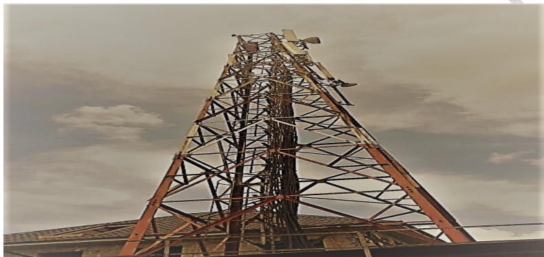
Figure 1. Picture of MTN Mast visited at Rumuolumeni
