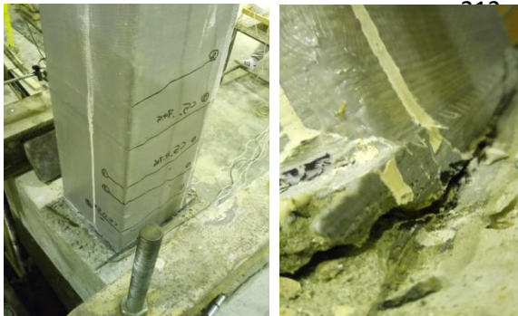
Figure 11: The cracks of C2G2 column at failure under the lateral load. Separation of the fiber is
