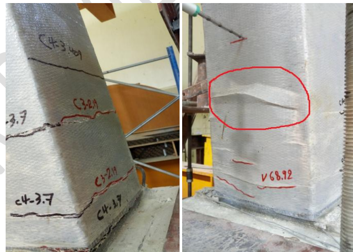
Figure 9: The cracks of C2G1 column at failure under the lateral load. Separation of the fiber is noticed.
