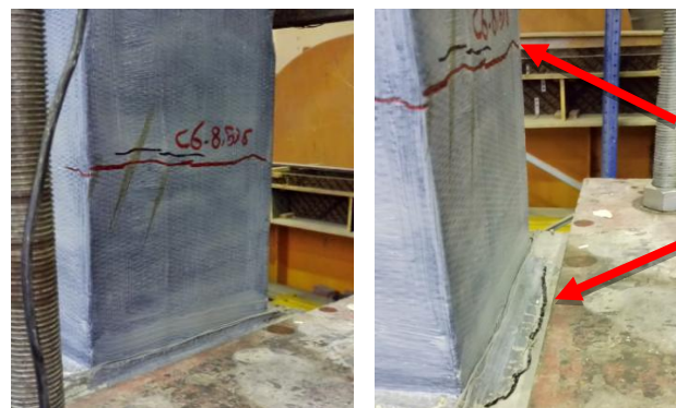
Figure 13: The cracks of C2C1 column at failure under the lateral load. Separation of the fiber is noticed
