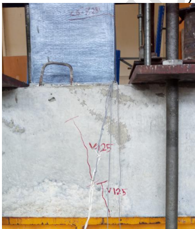
Figure 12: The cracks of column C2C1 at failure under the ultimate axial load
